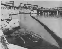
New floating rotary skimmer and floating boom are installed in the area of the Finger Piers.
